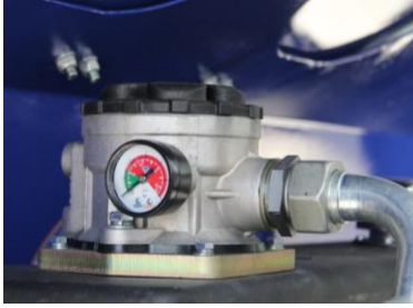
Filter Housing With Pressure Gauge
